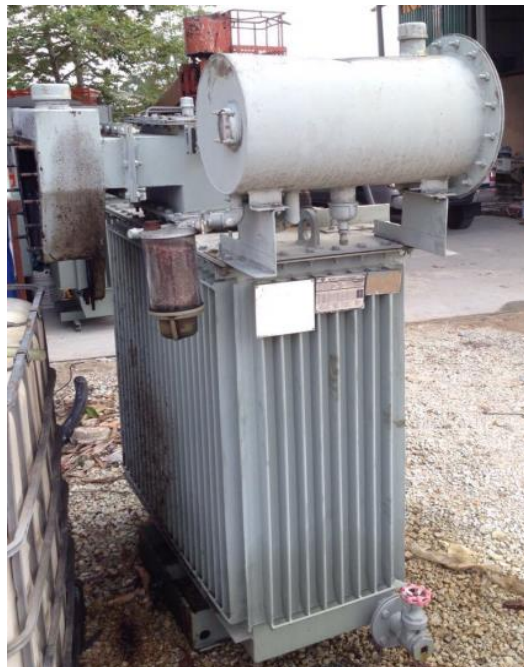
Figure 2. An In-Serviced Power Transformer
