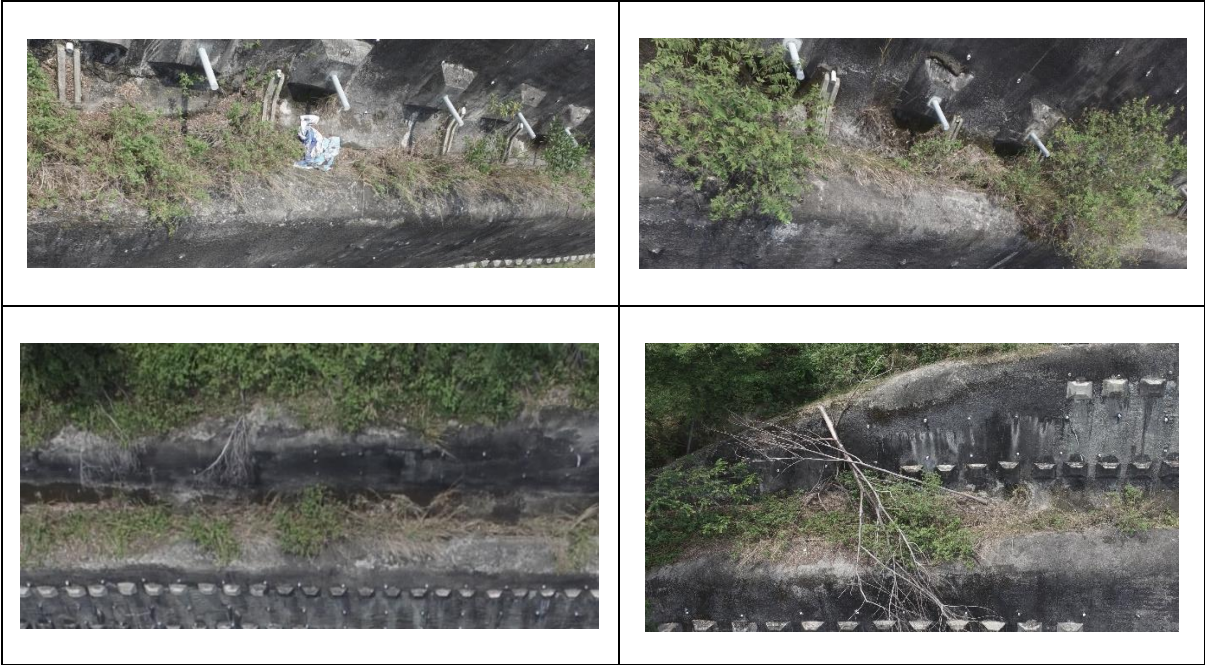
Figure 8. The excessive growth of vegetation in slope drainage at Jalan Kuala Pilah
