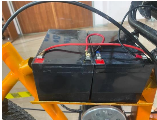
Figure 14. SLA 12V Batteries Connected in Series
